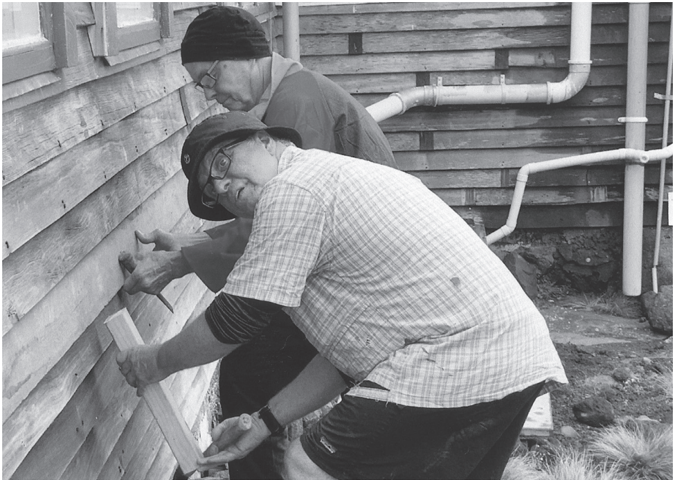
Simon Hunt and David Watt repairing weatherboards at the Lodge. Photo: Carl Burling.
